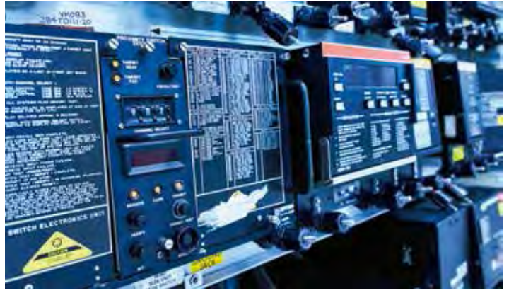
▶ Equipment in the dedicated computer room for the Boeing 767.
